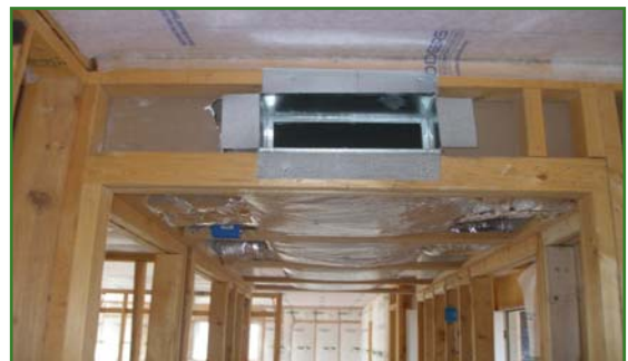
Duct work is sealed with mastic inside & outside all Seams
