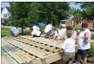
Teamwork! Frontier staff works together to complete a platform in Salt Lick
